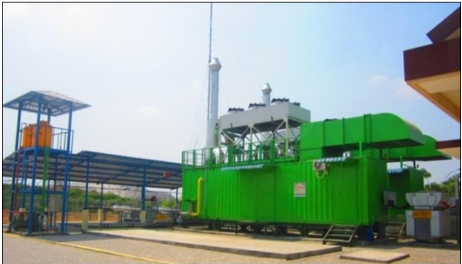
Gambar 4.4 Landfill Gas Power Plant di PLTSa Benowo
