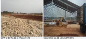
COW SHED No.11 at KALIATI SITE COW SHED No. 16 at KALIATI SITE
